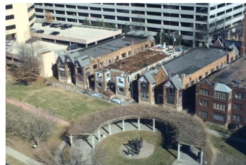
Nelle Peters apartments at 47 th and Summit mid-demolition, to be replaced by new residential construction
